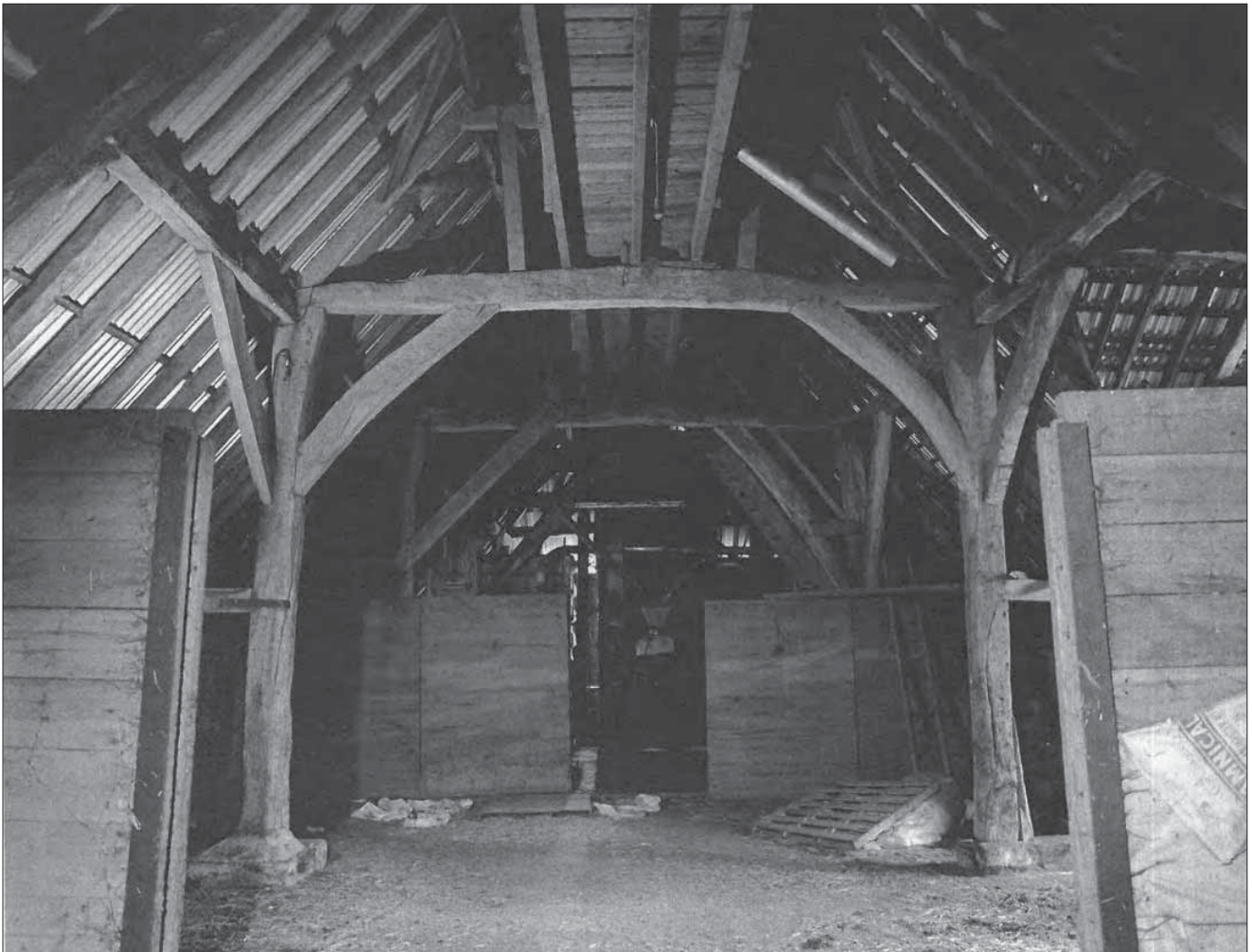
Appendix 4.13: Interior view of the southern barn from the east, taken in 2000. © English Heritage NMR Ref.: AA030291.
