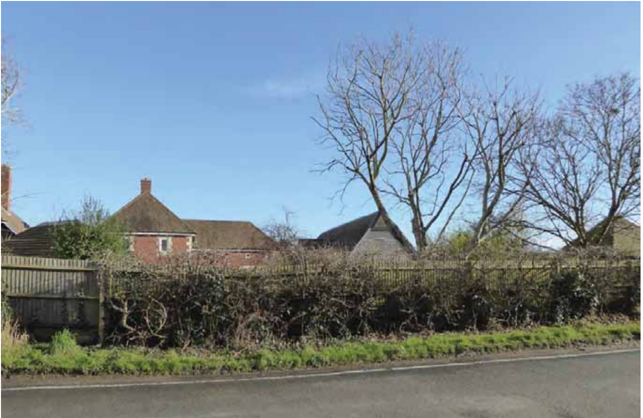
Appendix 8.3: The roof of the southern barn, from the north-west on Posbrook Lane.
